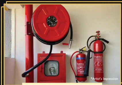
Fire Fighting System
