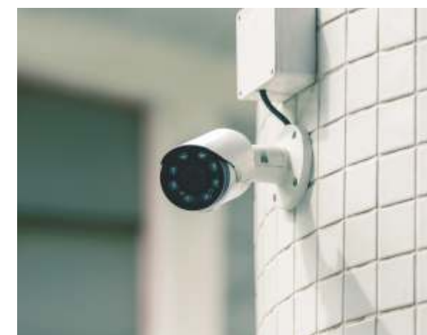
CCTV FOR COMMON AREAS.
