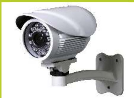
CCTV Surveillance in Lobby & Lifts
