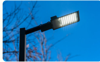
STREETLIGHTS ACROSS THE LAYOUT
