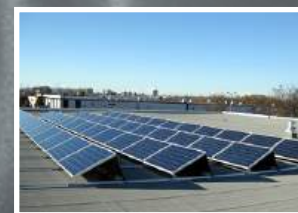
Solar-Power unit for common area
