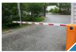
BARRIER GATE WITH AUTOMATIC SENSORS
