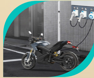
ELECTRIC VEHICLE CHARGING POINT
