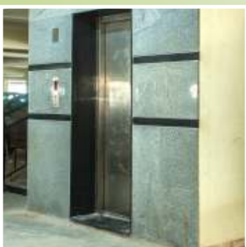
2 Lifts (Automatic with 6 passenger Capacity)
