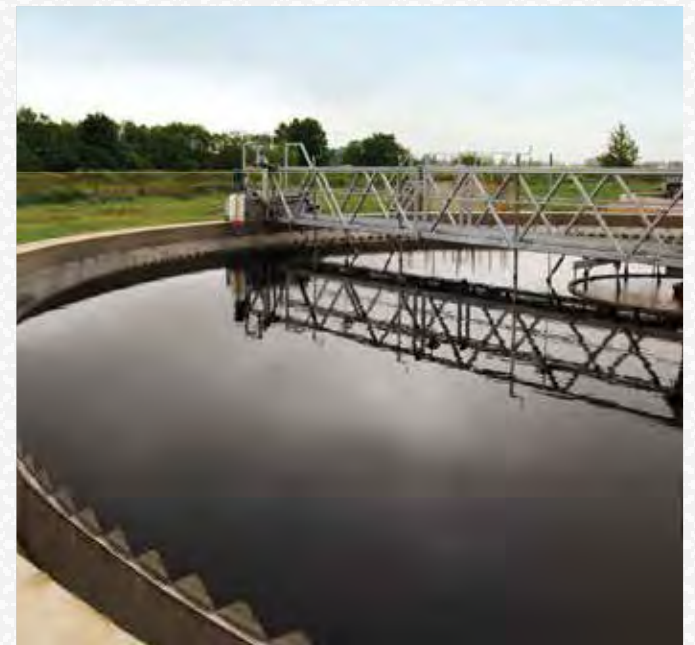
STP tank for waste water management
