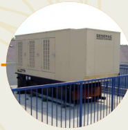
Power Backup for common area
