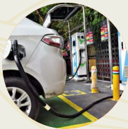
EV Charging Points
