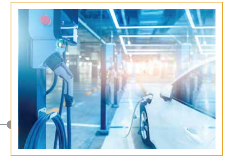
EV CHARGING FACILITY FOR EACH FLAT
