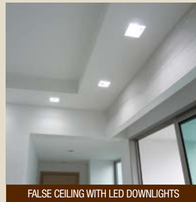
FALSE CEILING WITH LED DOWNLIGHTS
