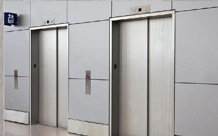
Two Lifts with 24 hr generator backup
