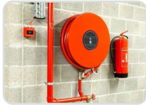
Fire Fighting System
