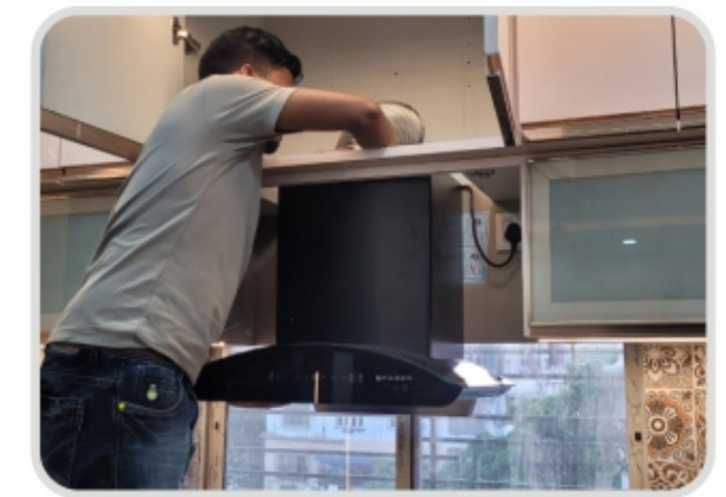
Kitchen Chimney Point
