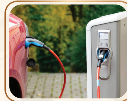
Electric Vehicle Charging Point
