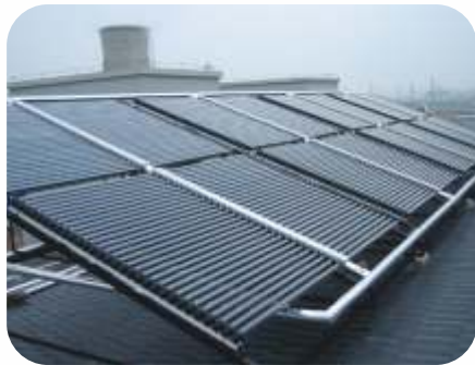
Solar Water Heater System
