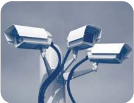
24x7 CCTV Camera
