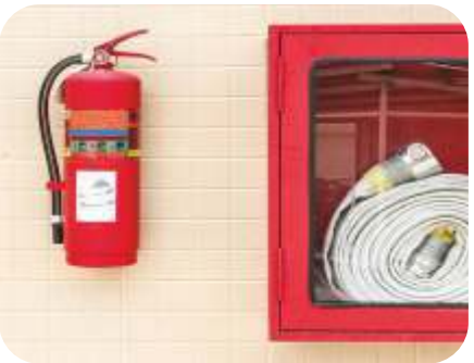
Fire Fighting System
