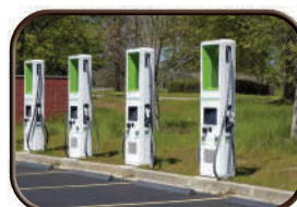
EV CHARGING POINT
