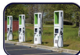
EV CHARGING POINT
