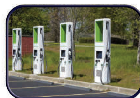
EV CHARGING POINT
