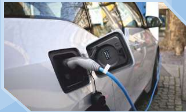
ELECTRIC CAR CHARGING POINTS
