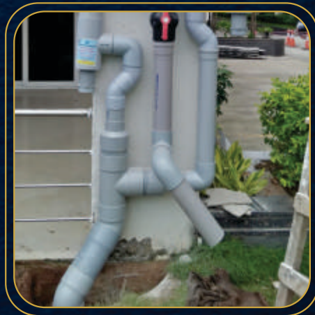
RAIN WATER HARVESTING
