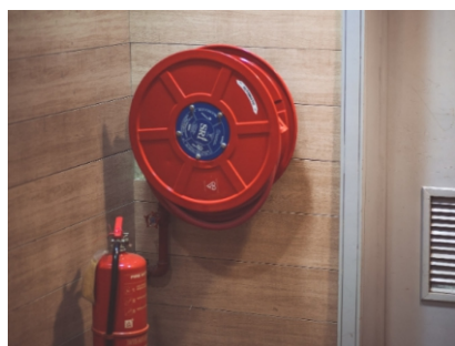
Fire Fighting System
