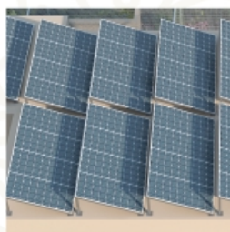
Solar Backup for Common Lights
