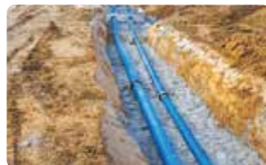
Underground Water Lines
