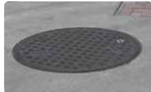
Underground Drainage System
