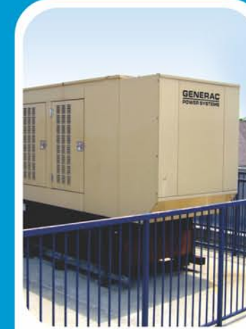
Power back up
