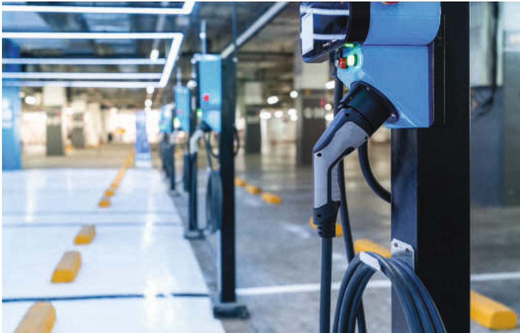
EV Charging Station
