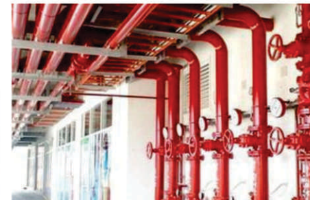
Fire Fighting System
