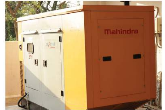
Power back up for common areas
