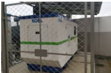
Power back up for Lift
