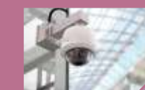
CCTV CAMERA SYSTEM
