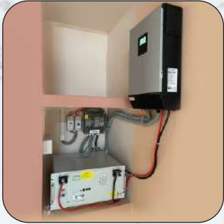
PROVISION FOR INVERTER
