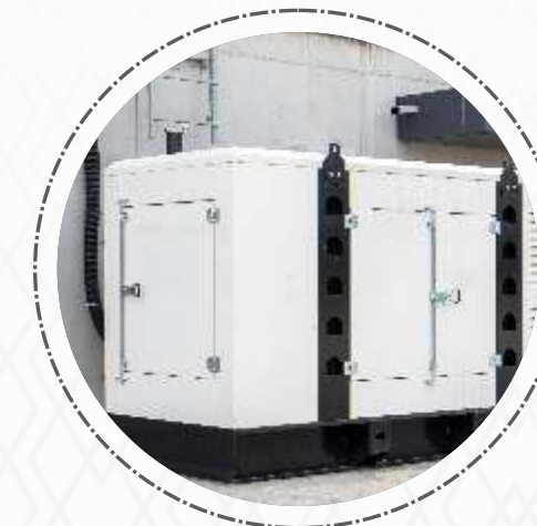
Generator backup for common areas
